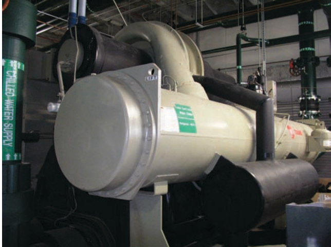
The Trane CenTraVac™ chillers at Cleveland Clinic Florida consume only .48 kW of electricity per ton of cooling capacity at full load.
