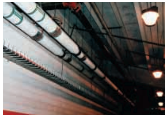
An expanded chilled water distribution system was installed to replace an earlier DX cooling system.
