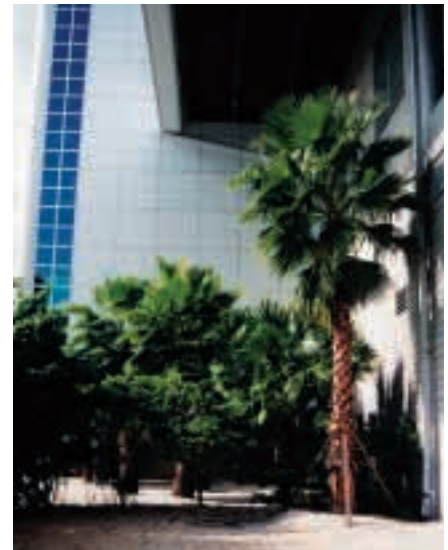
The area beneath the stadium overhang was formerly a source of heat buildup from the chiller fan discharge.
